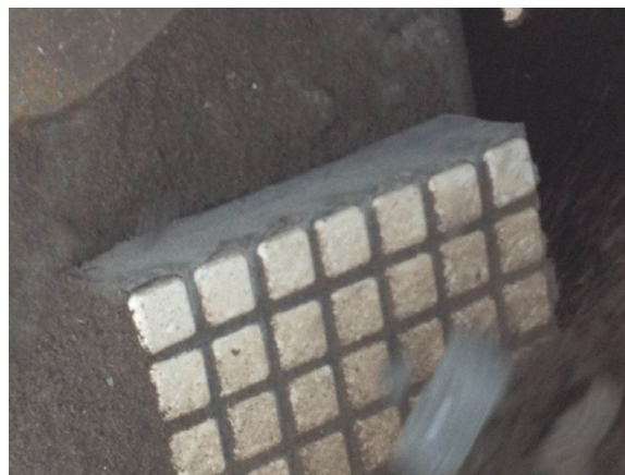
Redi-Liner Polyurethane in place at the bottom of the chute at the Hill View Quarries
