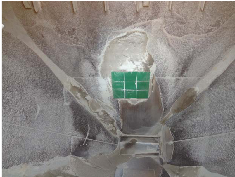
Redi-Liner Polyurethane in place at the bottom of the chute of St. Peters rail terminal
