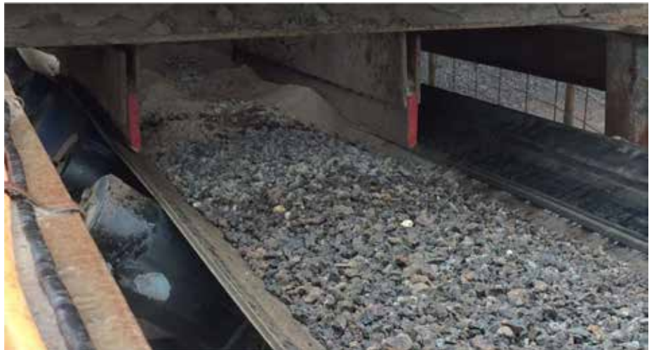
Close-up photo of the Argonics skirting installed on one of the conveyors at the transfer point.
